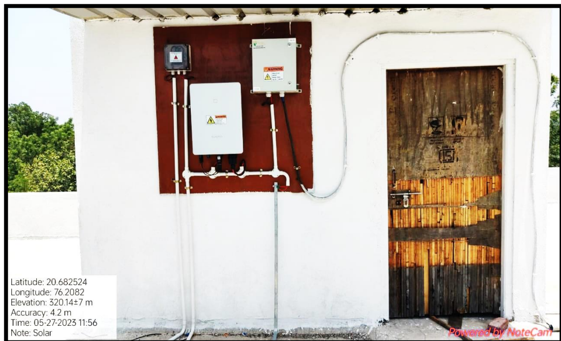
Solar Power System
