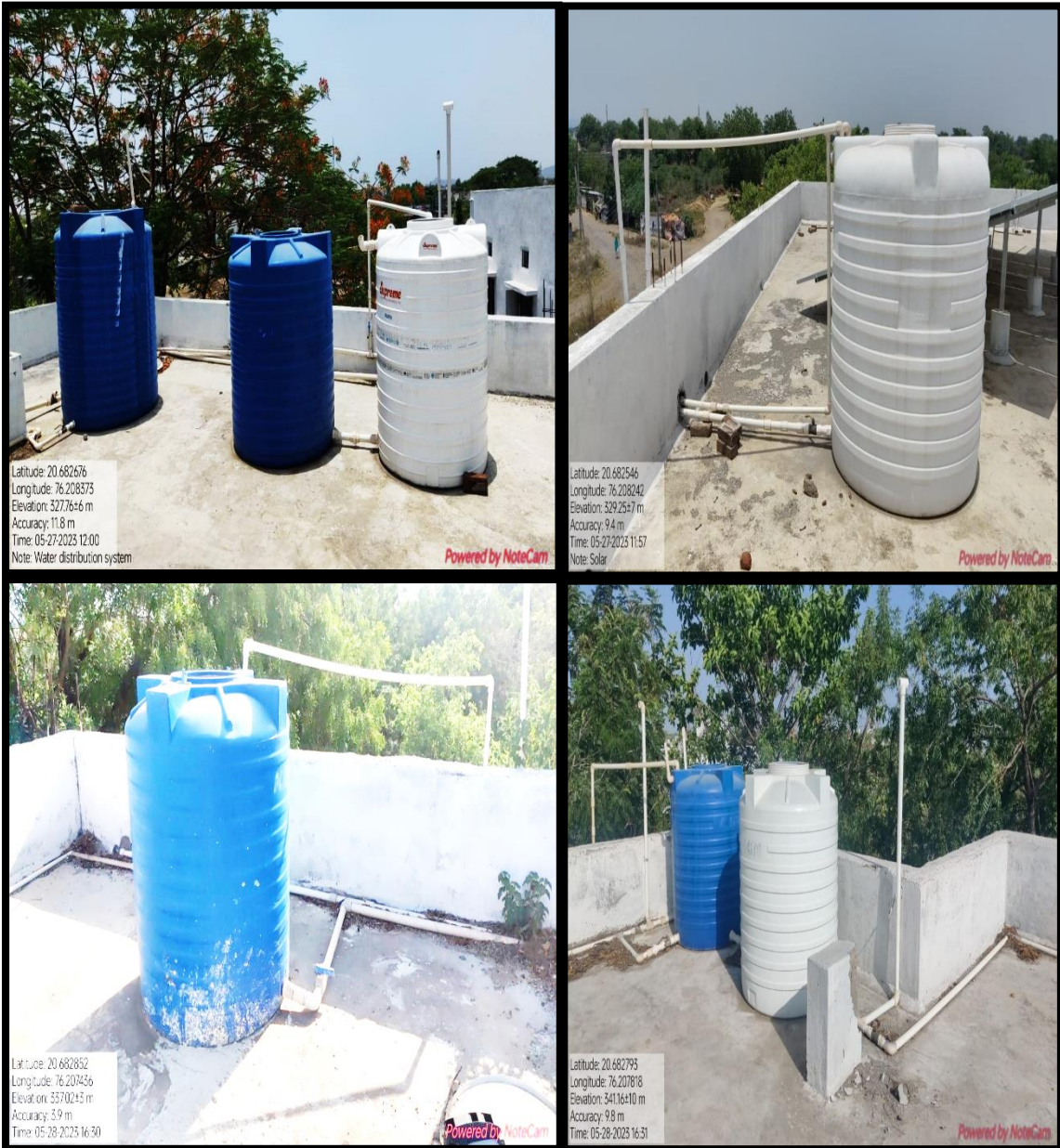
Water Distribution System at College
