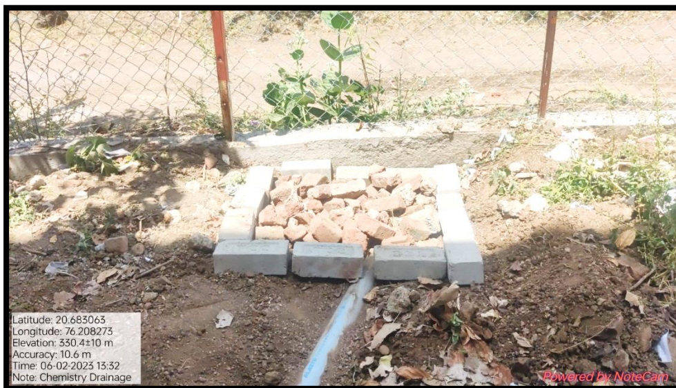
Drainage Pit of Waste Water of Chemistry department
