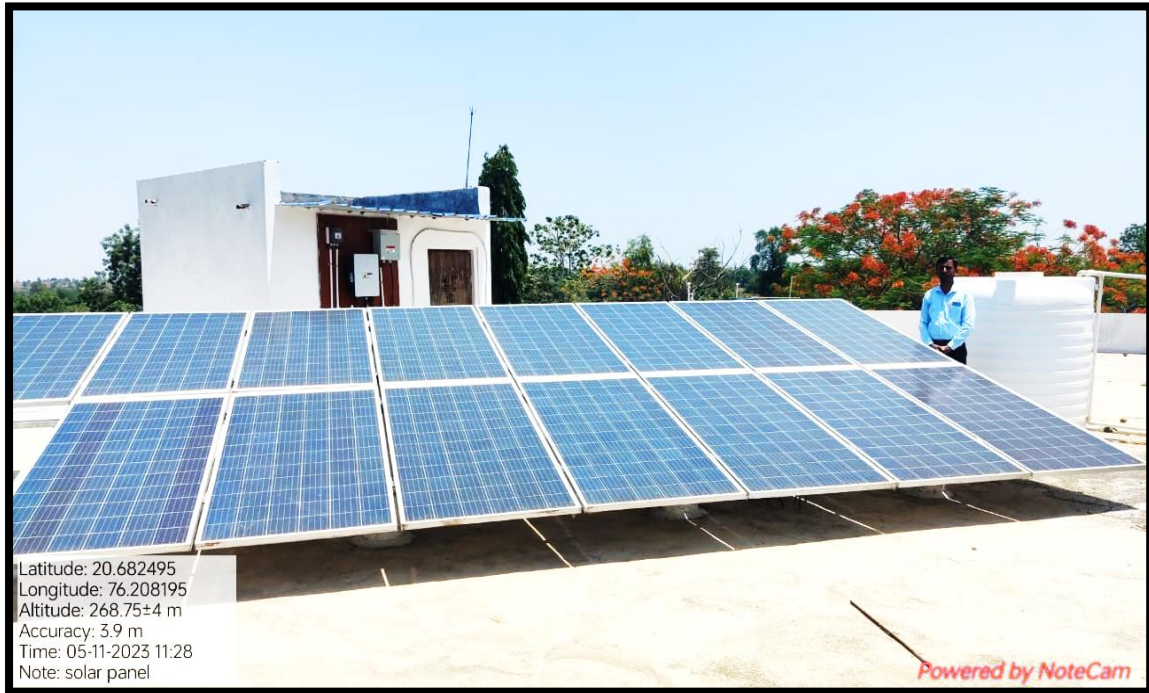
Solar Panel of 5 KW Installed at College
